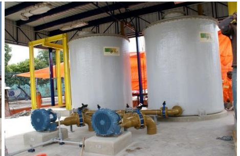
Compost biofilter for odor control
