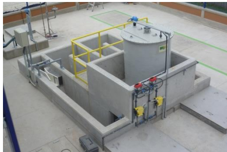
Contact tank with chlorine
